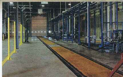
The rail car area, where raw material is delivered, is big enough to allow up to six railcars and four tanker trucks to be unloaded or loaded simultaneously.
